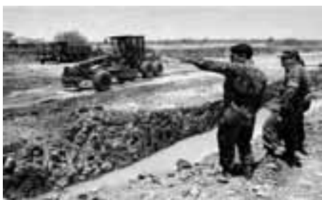
Soldiers stand guard as preliminary construction work is carried out in preparation for the transposition of the Rio São Francisco (2007)
